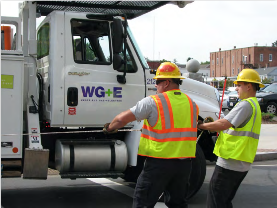
WG&E engineers pull fiber during network installation. Source: Westfield Gas & Electric/Whip City Fiber
